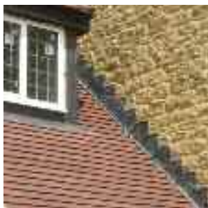
Multicourse Regular Wide Front to Back Dimensions. The natural hamstone is built against a concrete backing block resulting in an external leaf of 250mm thickness beyond which is the cavity. Thus the trays have extended front to back dimensions.
