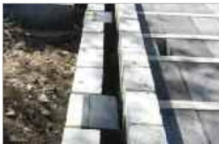
Telescopic adjustable ventilators (Type TAV) (to ventilate underfloor areas) have been built into the exterior cavity wall prior to bedding of the perimeter Cavicloak. Each ventilator has been extended in height to take advantage of the Cavicloak bedding level coinciding above it and providing protection. This approach removes the necessity to individually protect each ventilator at a lower course level.
