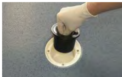
Lift out Trap using cross bar and rinse thoroughly.
