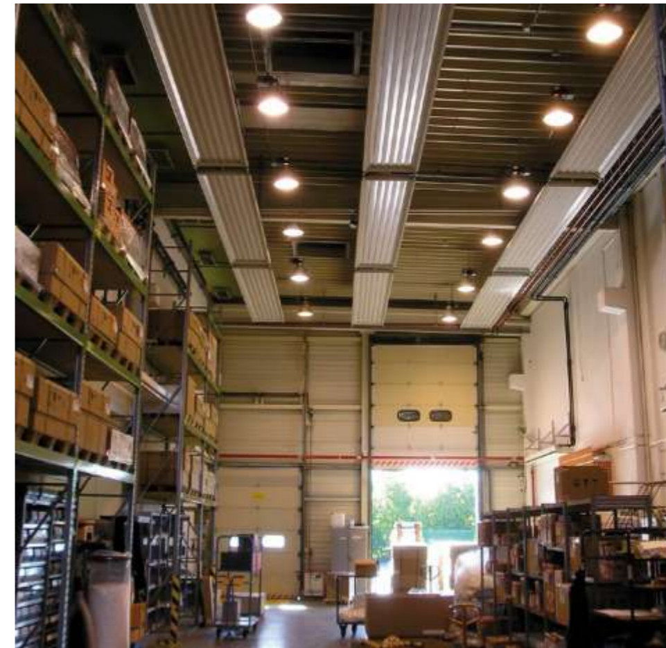
Strada Hi-Rad Plus in warehouse area
