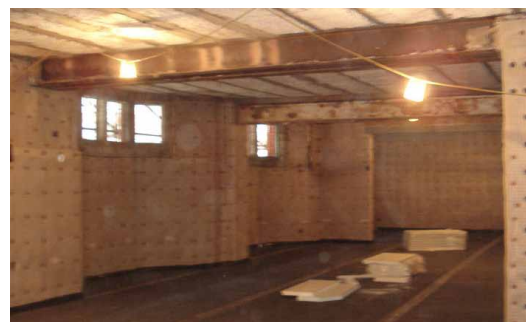
BBA approved cavity drain membrane Newton 508 Mesh was applied to the internal walls
