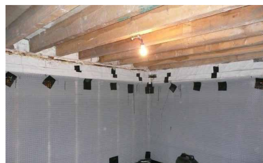
Installation of Newton PAC System, Newton Overtape used to seal around fixings to prevent gas leakage.
