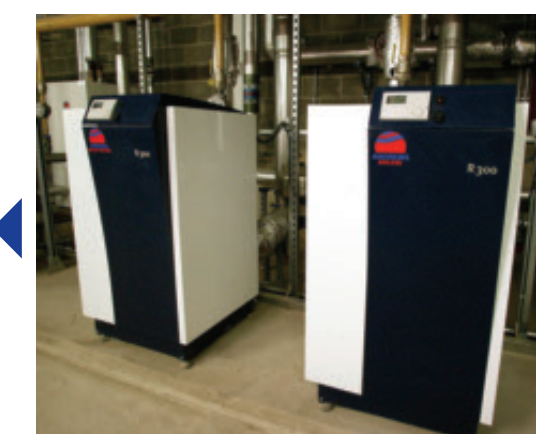
Two R300 water heaters at Little Sisters, Glasgow.
