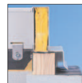
Existing Irregularly Sized Curbs
