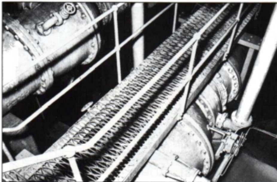
Two cylinder operated Larner-Johnson regulators, sizes 915 x 760 mm and 915 x 530 mm installed on a reservoir outlet for scour and supply control respectively. The cylinders are side mounted on the valve and operate by hydraulic oil maintained at the required pressure by means of an electrically driven pump unit with supply tank. Remote control of the regulators and associated wedge gate type isolating valves is from a console in the valve house at the top of the tower, where flow recording and electrical valve position indicators are also installed.
