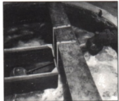
152mm inlet x 75 mm outlet Larner-Johnson Float Valve on inlet to break pressure tank. This valve was installed in 1932 and has given continuous service without attention (barring dismantling for inspection and cleaning on one occasion during alterations to the system).
