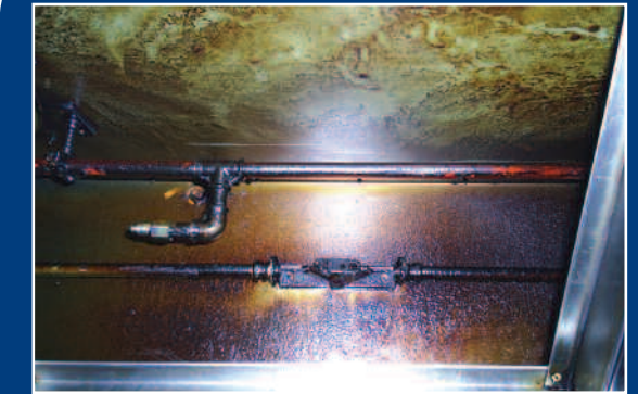
Without Ultrastream, grease can build up in the extract plenum and ductwork over a period of time, causing a significant health and fire risk. The plenum and extract ductwork system will require regular duct cleaning to minimise these risks.
