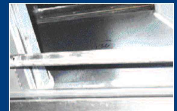
Ultrastream lamps remove grease and odours from the airstream. The above photograph shows a system that has been installed for 100 days and the primary filters have been removed. You can clearly see the plenum is clean and free from grease.
