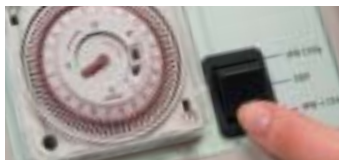
Switch to electric hot water and heating
