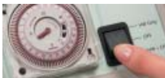
Switch to electric hot water
