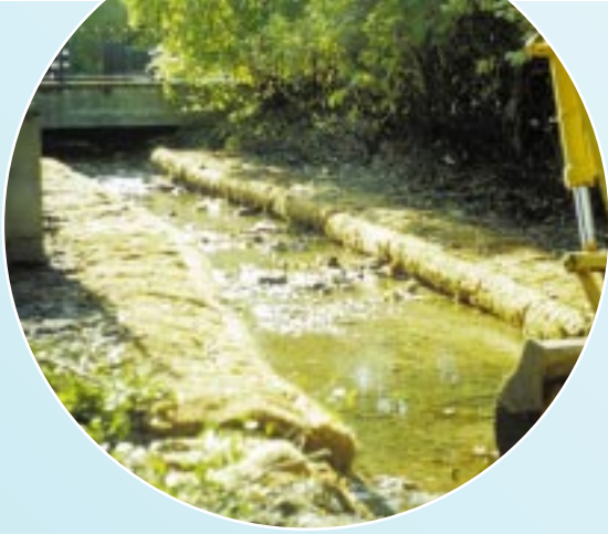
Sainsburys, Sevenoaks using Bio-pallets and Bio-rolls to establish vegetation and control sediment build up.
