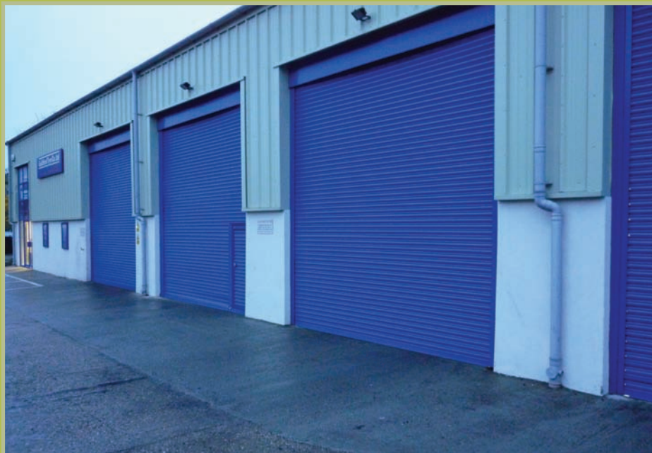
Harling HS75 steel shutters, powdercoated, with a wicket access door installed with 3 phase motors.
