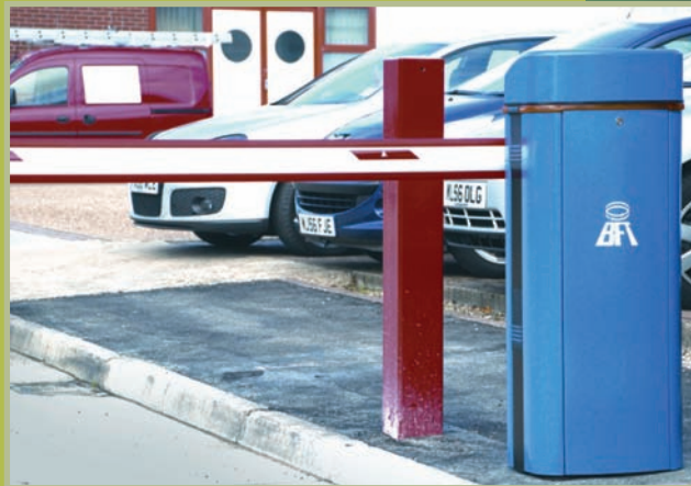
Automated barrier with a steel protective post to one side
