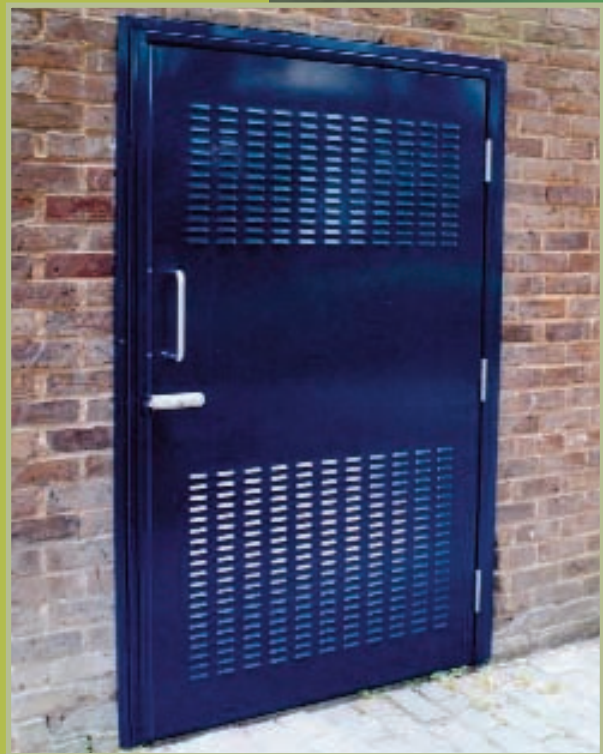
Vented HS Raidor substation door
