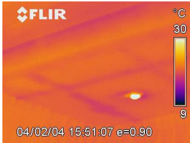
Moisture tracking along battens above a ceiling.
