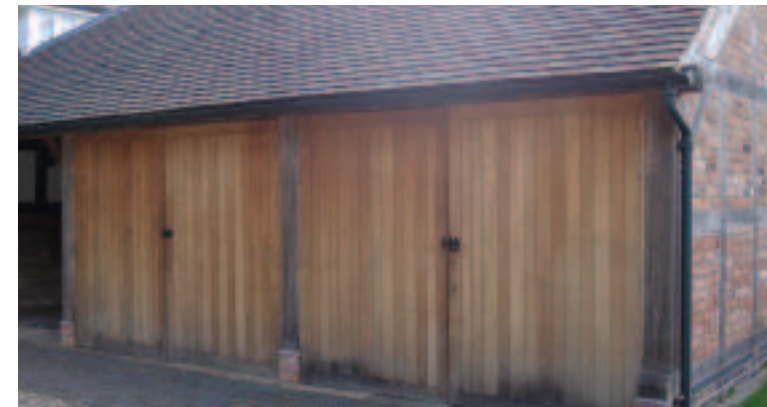
double garage doors (weathered)
