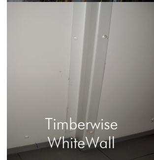
Electrics on damp wall
