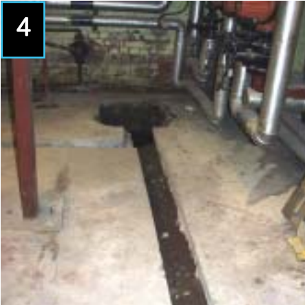
Mid-floor chases are cut out, ready for TrenchDrain™ (ACO), and a hole excavated for one of the sump locations.
