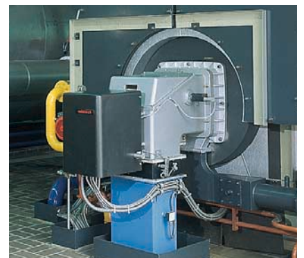
WKGL50 dual fuel burner in operation
