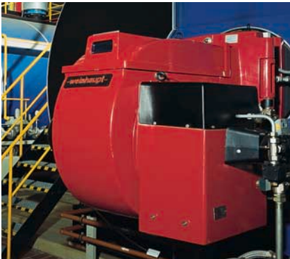
RGL70 dual fuel burner in a heating centre
