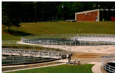
Wastewater treatment operations
