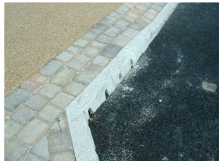
ACO KerbDrain installed – Finish of the product tailored to colour match surrounding environment.
