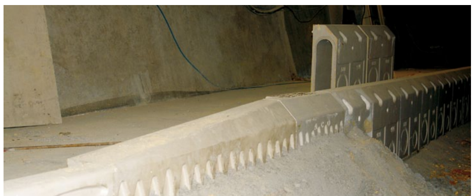
Drop and centre stones at tunnel link passage carry the splay profile to the finished road level.
