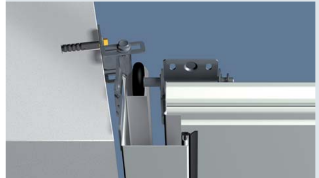
Chamfered and uneven side wall
