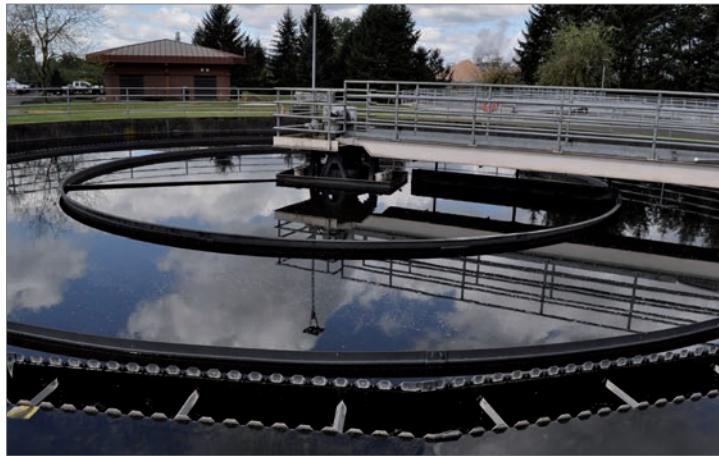
Primary clarification system
