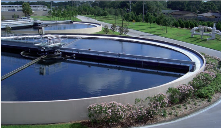
Large primary clarifiers
