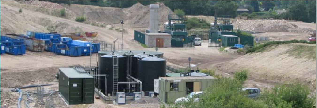
Figure 1 Beacon Hill landfill site leachate treatment plant
