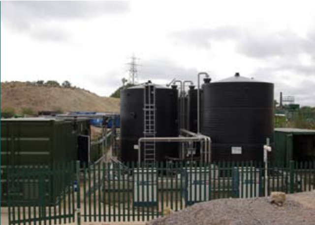
Figure 2 COD and ammonia is treated in three bioreactor tanks
