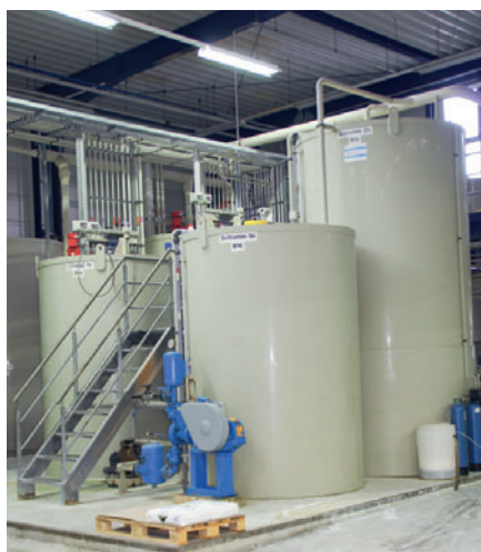
Separation of zinc and nickel
