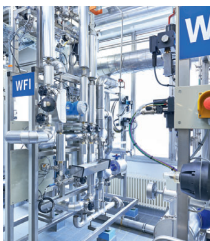
WFI storage and distribution system. Source: SH+E GROUP
