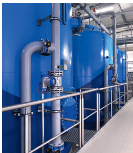
Water softening plant
