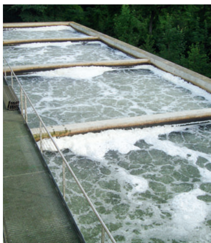
Activated sludge basin for fixed bed filtration
