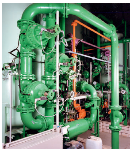
Power station water treatment
