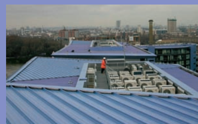
View of a Bilco D-50 REM smoke vent from the rooftops with H&V equipment alongside.
