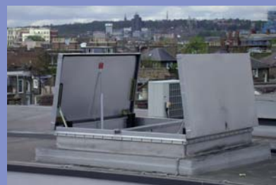
Double leaf smoke vent in fully open position.
