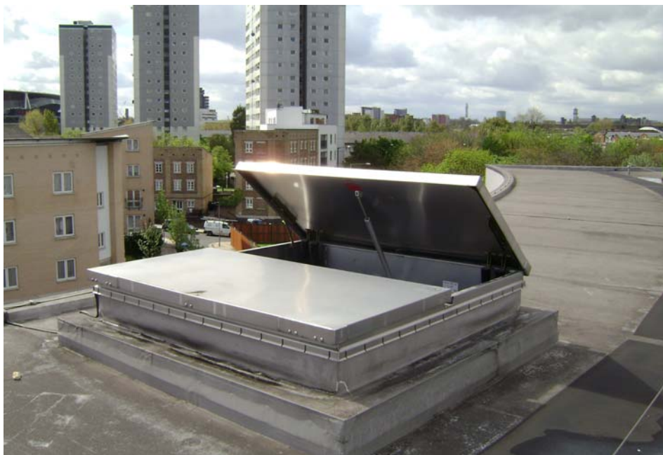
The Bilco smoke vent on the roof at the Medical Foundation for the Care of Victims of Torture in London.
