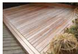
Q-Deck® Lyptus showing early signs of weathering.
