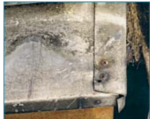
Steel rivets in mill finish aluminium after 24 years exposure in an urban atmosphere.
