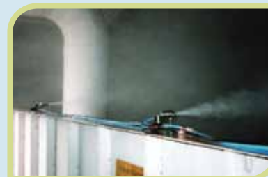
Treatment of residual odours from bio-filter
