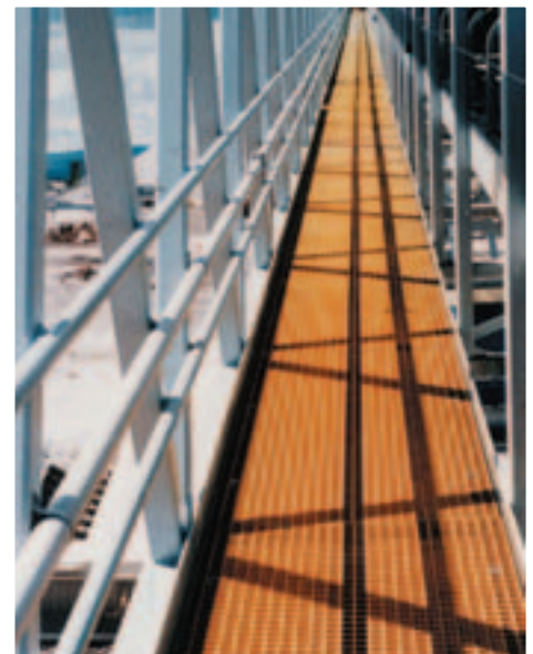
Fibreglass Grating walkway at salt works
