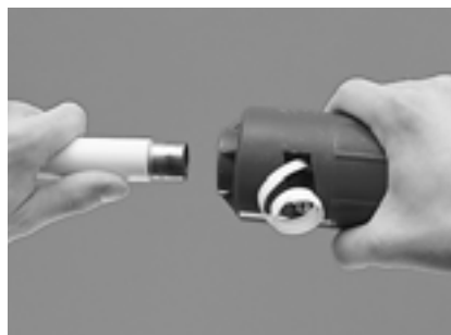
Figure 8.0-28 Stripped mapress CARBON STEEL pipe
