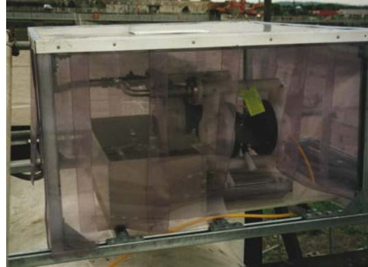
Air operated Dosing Pumps, with stainless steel pipework and Polypropylene Bund
