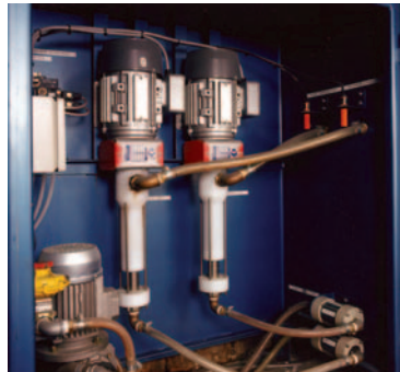
2 LF pumps delivering sulphuric and sulphonic acid at a steady and consistent flow
